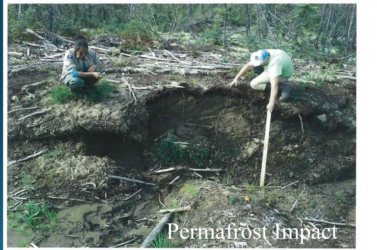
Ground view of trench 3 miles south of FGH (N66 15.295, W128 32.010) showing extent of erosion; trench depth is greater than 4 feet (length of pole) and wider than 8ft at spots. The cable is exposed and hovering taught 1 ft above the bottom of the trench.
