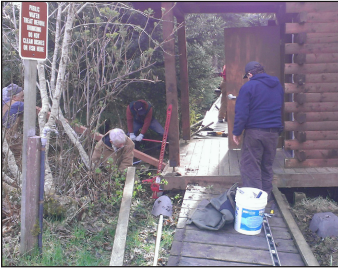
Friends of Kachemak Bay State Park level an outhouse lifted by the freeze thaw cycle.
