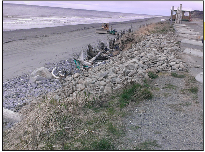
Anchor Point community members pulled together to repair an eroded grade and save the parking area for a local tractor launch from collapse in Anchor River State Recreation Area.
