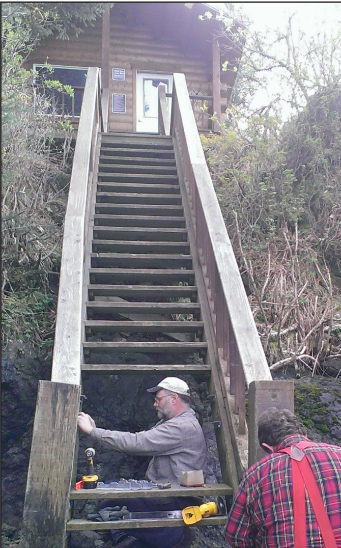
Friends of Kachemak Bay State Park repair old stair treads for the Halibut Cove public-use cabin. Just a few more to go!
