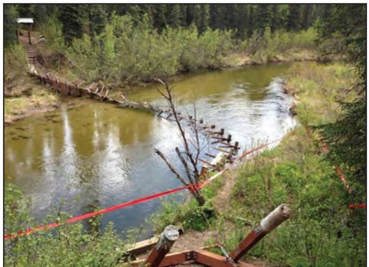
Byers Creek Bridge collapsed this spring.
