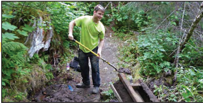
ACC Matthew Fatuch digs a trench to improve drainage along the trail.
