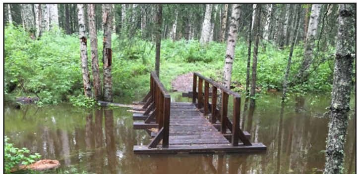
The bridge along the Rosehip Nature Trail in Chena River SRA became a floating bridge. Luckily, the bridge is cabled and only had to be moved a short distance for re-attachment.
