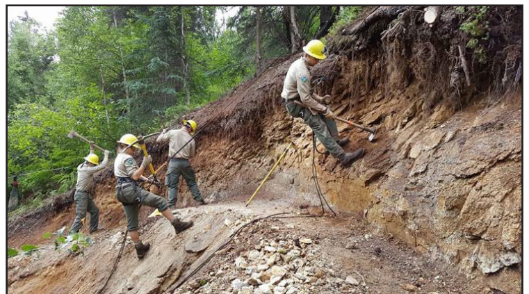
This section of trail slid into Troublesome Creek 50 feet below, causing the trail crew to have to cut new trail tread into a granite rock face. Safety lines and rigging was expertly established and supervised by Park Specialist Justin Diapola-Allen (not pictured). Another DSP project completed in a timely manner and without injury or incident! (L-R) ACCs Ryan Johnson, Gemma Amorelli, Liam Jones, and Riley Bickford
