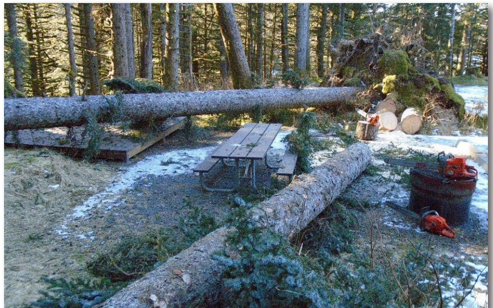
Work is underway to clean up fallen spruce trees in the Fort Abercrombie State Historical Park campground after a windstorm.
