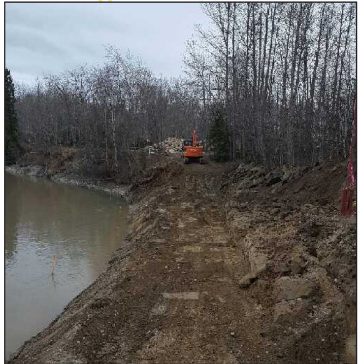
The bank stabilization project at Big Delta State Historical Park is underway. The project will protect four historic structures threatened by the Tanana River. Funding for the project came from a variety of private foundations, local businesses, and the federal Historic Preservation Fund program.
