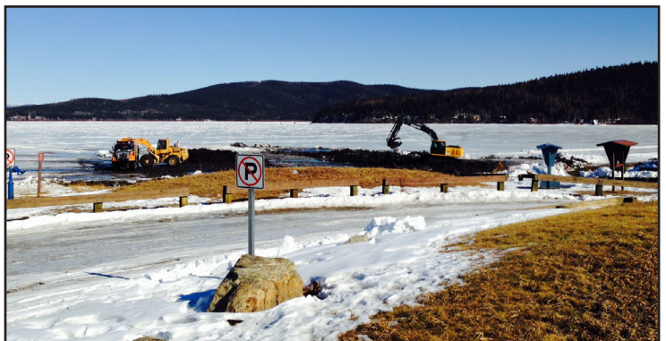
The boat channel at Quartz Lake SRA was dredged the first week of April. Close to 2,000 yards of sediment were removed, allowing boaters smooth access to the lake and saving them money on props and shear pins come summer.
